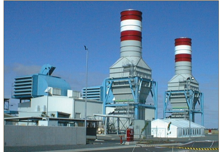
Oakey Power Station
